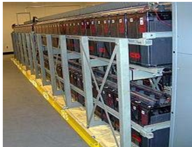
Figure 2 – A bank of batteries in a large data center, used to provide power until diesel generators can start
