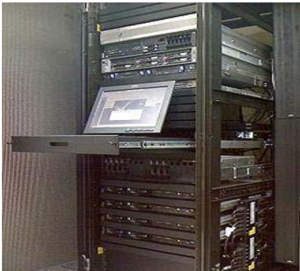
Figure 1- A typical server rack
