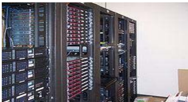
Figure 3. - Multiple racks of servers, and how a data center commonly looks.
