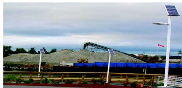
Fig. 2. CFL with stand alone lighting system for surface mine haul roads
