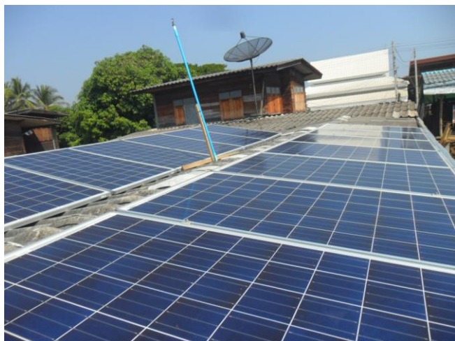
Fig. 1. View of the 3.5kWp rooftop PV plant.
