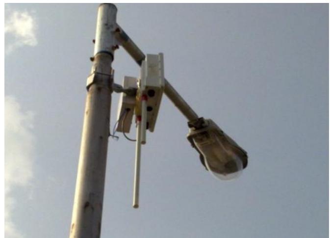
Fig. 3(b) Mesh Point mounted on street pole
